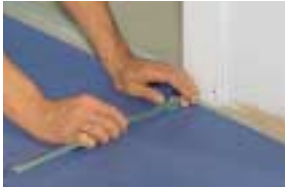
Trace the shape of a doorpost to the linoleum with the help of a scribing bar.
