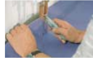
The loosely-laid sheets are cut in, around a radiator in this case, after ensuring the subfloor is flat and smooth.
