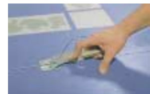
The weld rod is trimmed in two operations, first with the trimming guide fitted, then with the bare blade.
