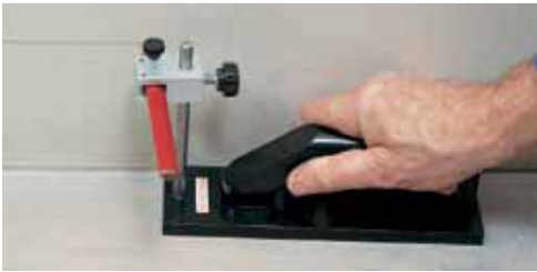
Fix the profiles following the adhesive manufacturer's instructions. Mark in pencil the height of the vinyl skirting on the walls.
